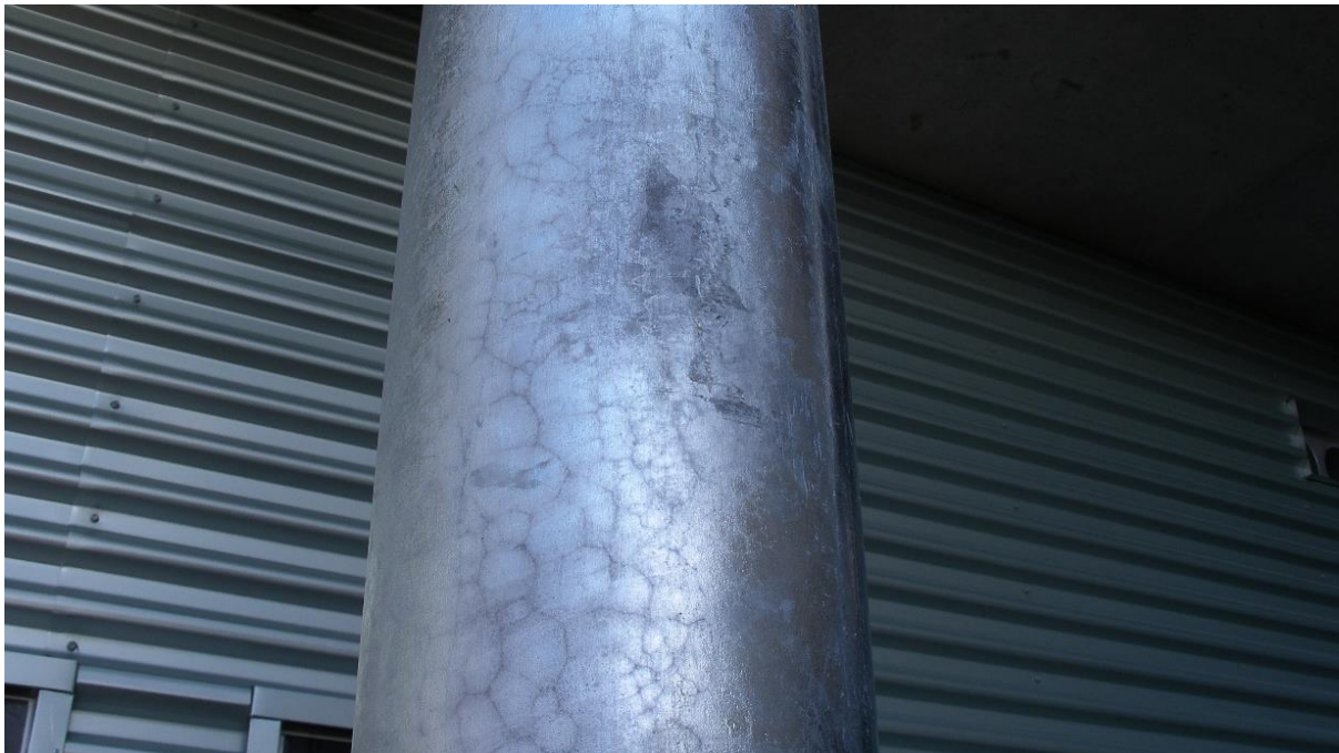
Figure 3: Mottled appearance on a pipe, most likely due to the steel chemistry.
