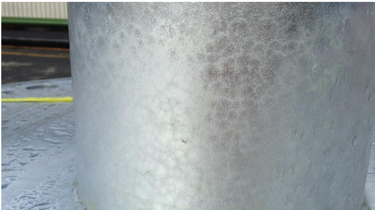
Figure 4: The scale like mottled appearance evident on a circular article.
