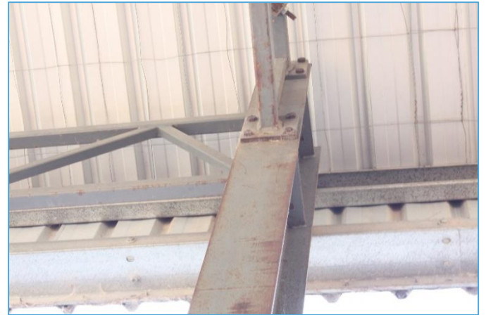
Above: The same sun-shelter as on the left, showing the in-line galvanized purlins with the coating performing well, even though they are rain sheltered.
