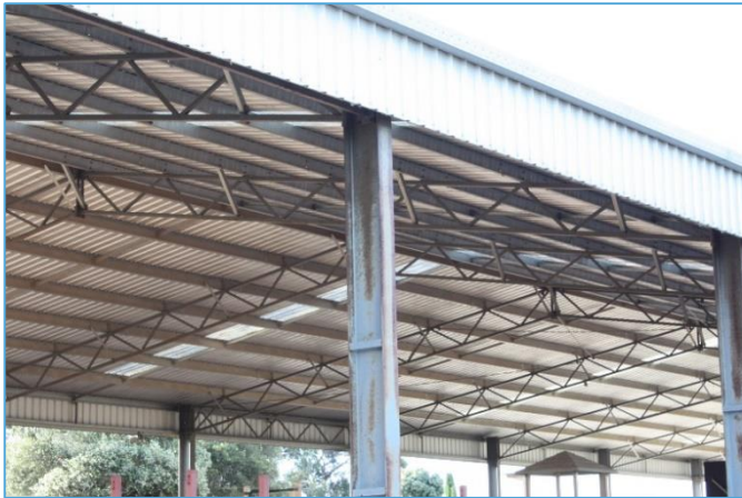
Above: Breakdown of the single coat paint system in a low corrosivity environment (C2) on a large sun-shelter located in Tatura, Victoria.
