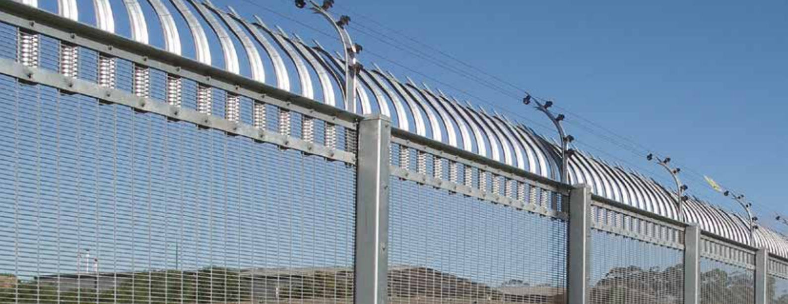
Electrical Sub-Station Fencing
