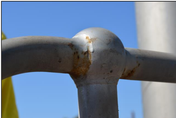
An example of poorly repaired handrail in a severe corrosive environment (wastewater treatment plant) where the repaired area has failed well before the main hot dip galvanized rails and posts.
